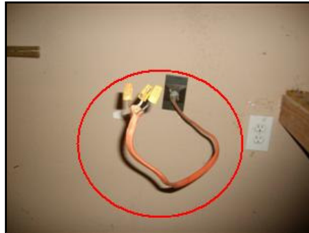
2.0 Picture 2 Disabled Circuit
