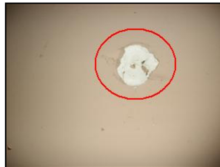
1.0 Picture 4 Sheetrock Defects
