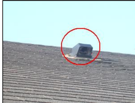
1.0 Picture 2 Dryer Vent
