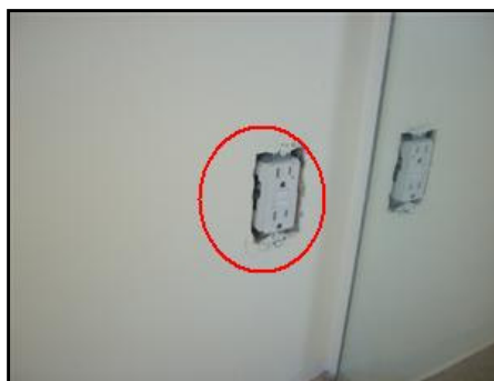
2.0 Picture 10 Missing Cover
