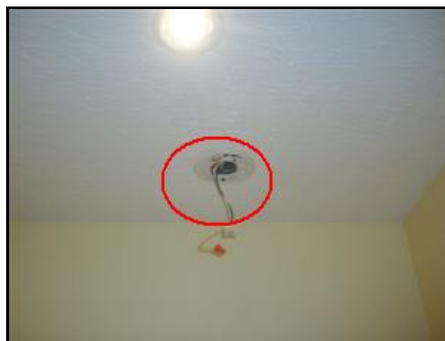
2.0 Picture 8 Missing Smoke Detector
