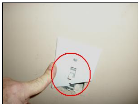
2.0 Picture 9 Broken Cover
