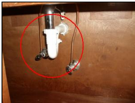
9.0 Picture 1 Master Bath Drain is Stopped up
