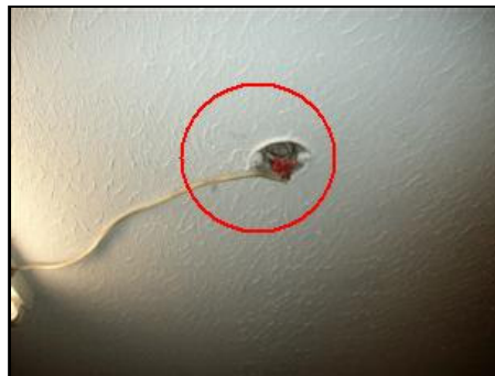
2.0 Picture 4 Open Electrical Box
